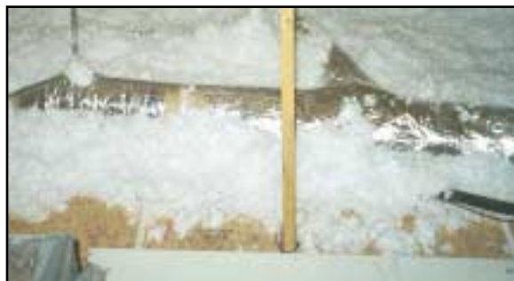
Insulation is piled up against the ducts to provide extra protection from the attic's temperatures.
