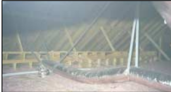
Suspended flex ducts droop between supports. The supports can restrict the air flow.
