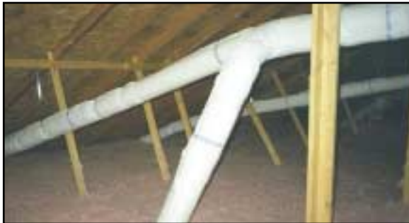
Suspended ducts are vulnerable to attic temperatures.
