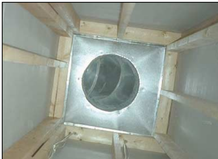
A home-made return air "duct." Note the unsealed electrical penetrations at the top that can pull down attic air into the return
