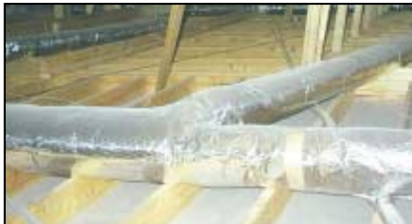
Metal ducts, sealed with mastic, are placed 2 inches above the rafters.
