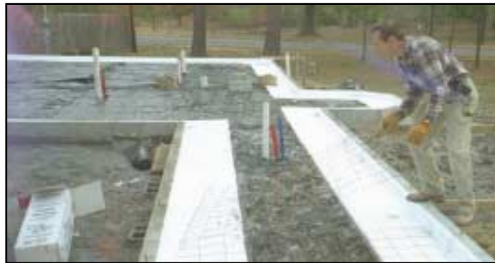
The remaining 20 inch piece is pressed against it on the ground that is covered with plastic sheeting. Over this is placed the welded wire mesh. Note also that the placement of the foam around the edge acts to absorb slab expansion and contraction.
