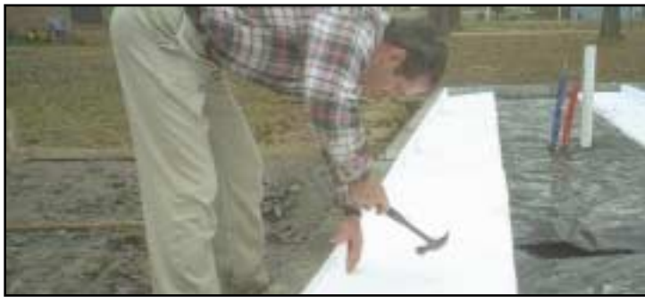
The critical top 4 inch piece of foam is placed against or nailed with 2 inch concrete nails to the solid "L" blocks.
