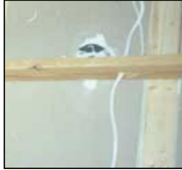
An unsealed light wiring box
