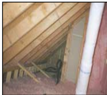
Missing knee wall insulation. Check the work.
