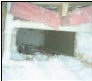
Hole in ceiling exposes many walls to attic temperature.
