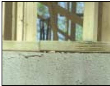
A leaking bottom plate
