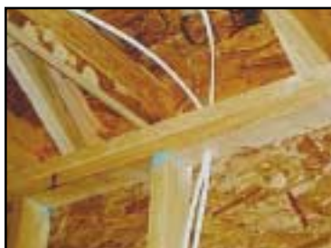
Wiring penetration in top plate is open to attic.
