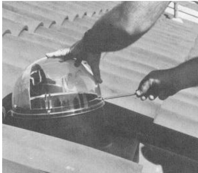
Figure 3 -- The clear acrylic dome is installed with the internal "scoop" facing south to capture maximum sunlight.
