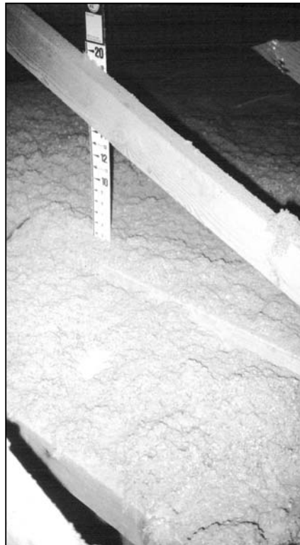
Depth gauges are no guarantee of quality if an installer ignores it, as happened in this attic.
