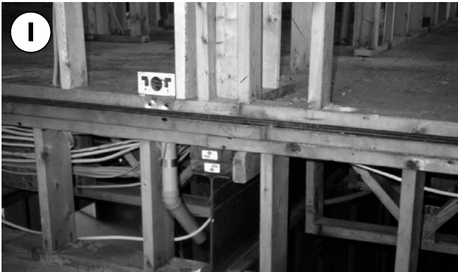
Before the garage is Sheetrocked, it is easy to see that this floor system is open to the garage. Without proper sealing, car exhaust and fumes from stored chemicals can seep directly into the house.
