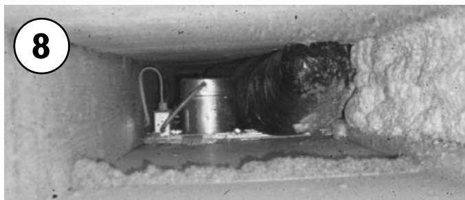
Often when the insulation is removed, you can see from one side of the house to the other. When this is the case, the floor space, and the plumbing pipes, ductwork, and lighting inside the floor, are now in the attic. They are exposed to the extreme temperatures of the attic.
