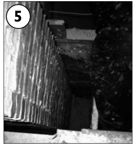
Standing in the attic, one can look into the chimney chase and down into the house. When this cavity is heated, the air rises into the attic, turning the shaft into a chimney for the house's conditioned air.
