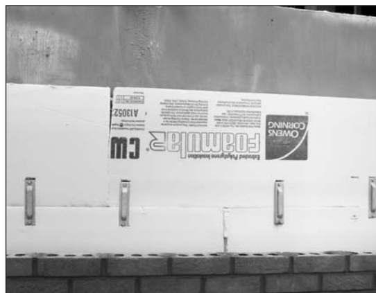
This rigid foam might be on the edge between Grade I and Grade II; notice that the mason had inserted a small piece of foam to fill part of a larger gap (lower center). There are more gaps and skewed pieces nearby at the exterior corners (outside the photo), so this ends up as a Grade II.
