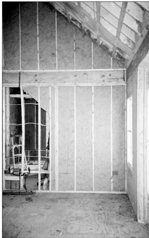
This sprayed cellulose job is a Grade I for sure—filling all cavities completely, firm to the touch, and not slumping away from the top plates.
