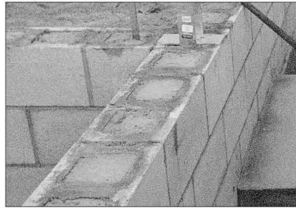
CMU cells filled with grout shrink, creating termite highways to the floor structure. The cells must be sealed with Pro Poxy or a similar sealant.
