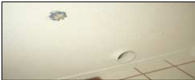
This is an excellent example of a finished dryer vent and water shut-off valve.
