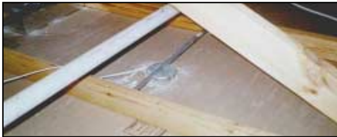
Before the ceiling is insulated, caulk around all holes that were made through the sheetrock.
