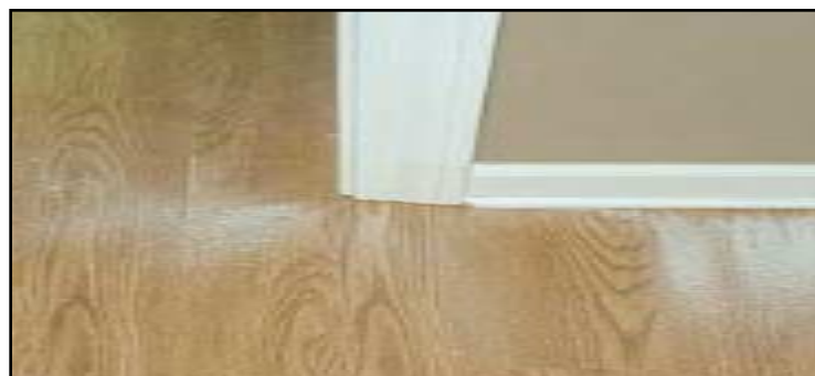
Evidence of a leaky interior wall.
