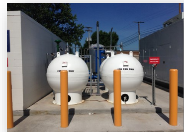
CNG storage tanks at CATA CNG station.
